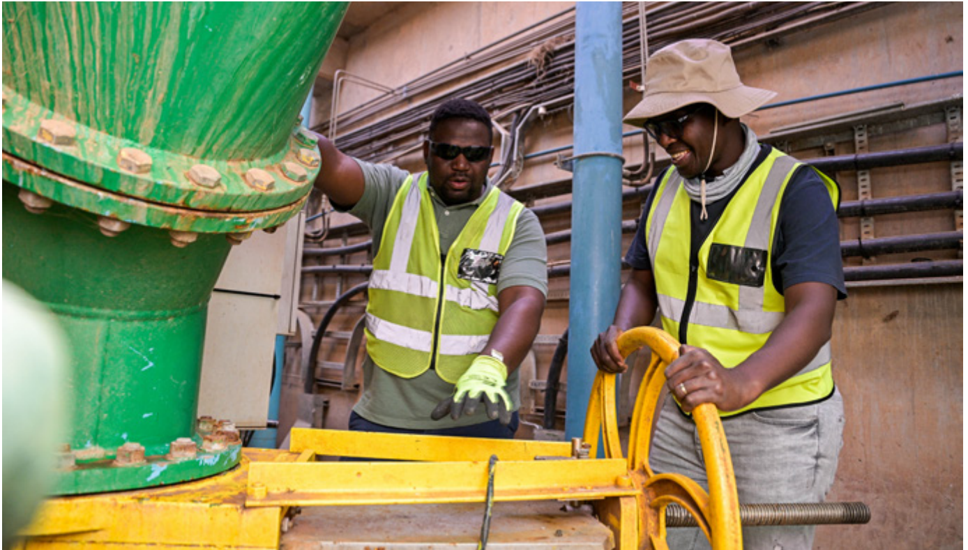
📷 Collins Monareng, Fitter, and Khutso Sihlangu, Head of Engineering and Reliability, inside the Havercroft Weir
