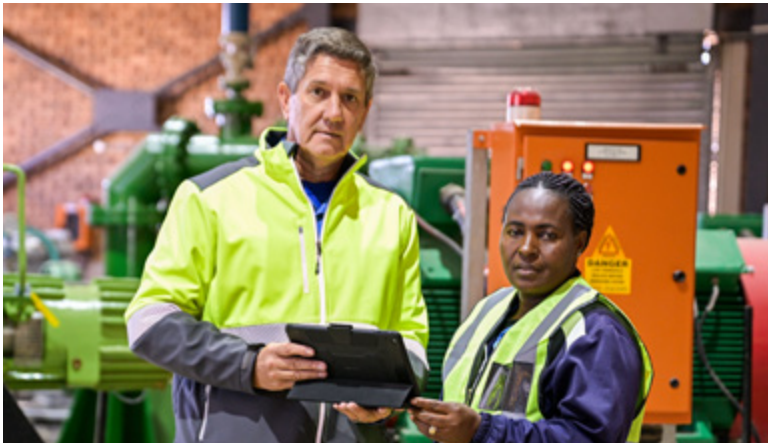
📷 Willem van Aswegen, SHERQ Manager, and Hanna Shai, Safety Officer / Coordinator, at Spitskop Pump Station 2.
