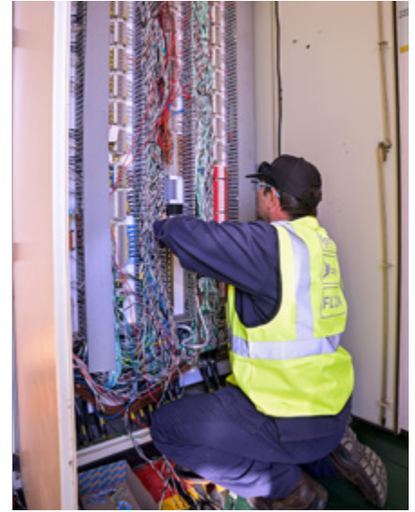
📷 Wiring check, Clapham Pump Station.
