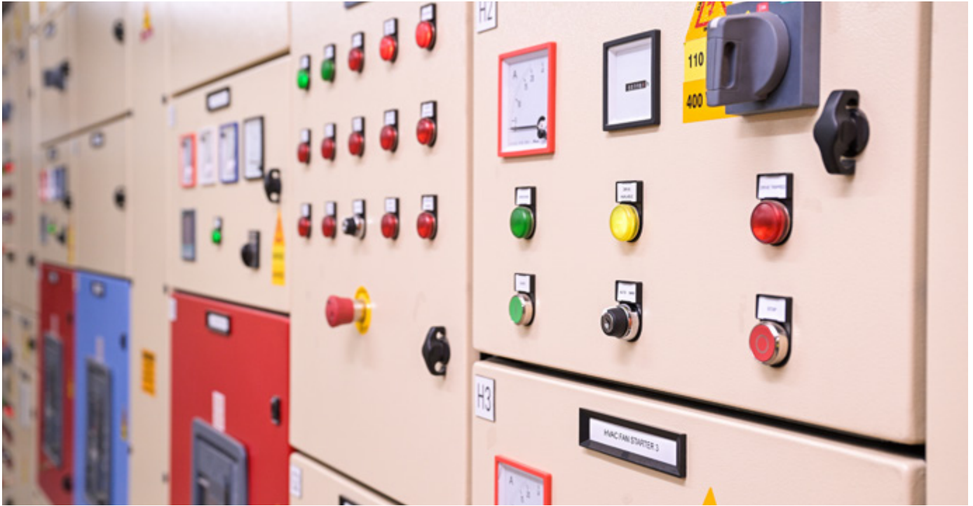
📷 Control room in Spitskop Pump Station 2.
