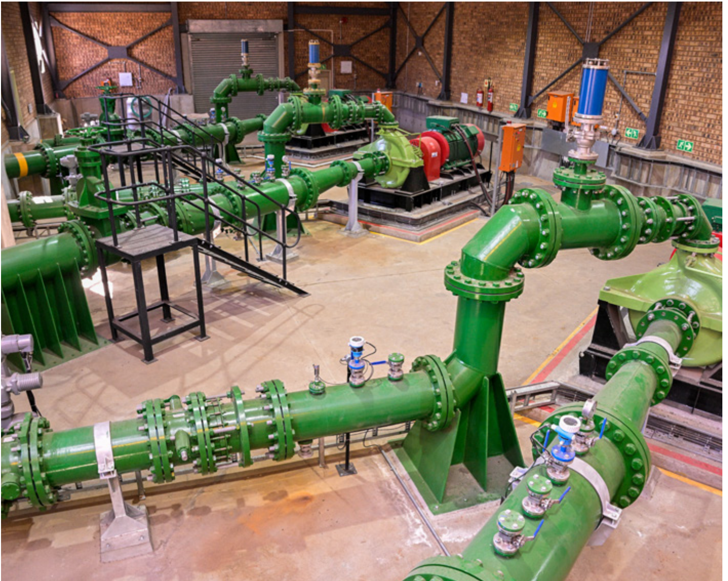
Spitskop Pump Station 2.
